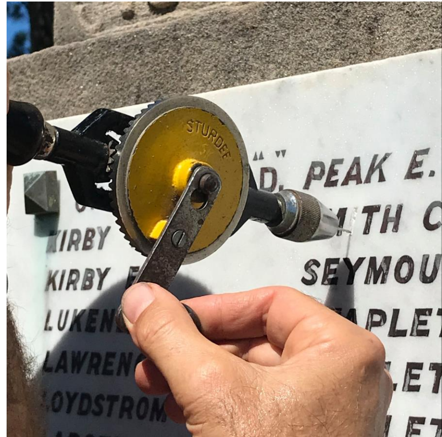
Specialist repairs to the lead lettering on the Woy Woy War Memorial Photo supplied by the Merril Jackson
