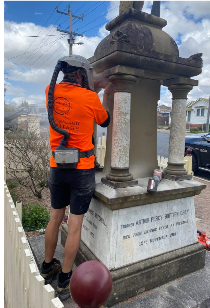
Conservation work being undertaken to the Tenterfield Boer War Memorial. Photo supplied by the Tenterfield RSL sub-Branch
